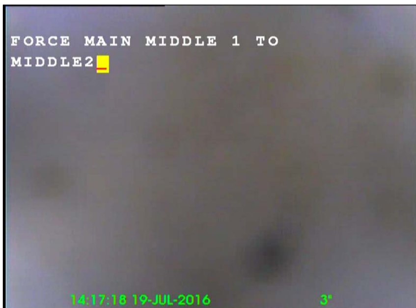
Photo: 3_3_13_A.jpg 0.3FT, Water Level, 40 %of cross sectional area
