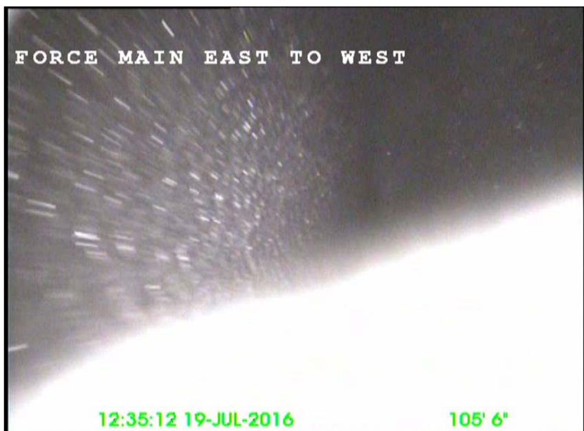
Photo: 1_1_8_A.jpg 105.6FT, Water Level, 5 %of cross sectional area
