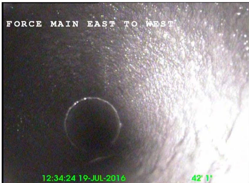
Photo: 1_1_6_A.jpg 42.5FT, Water Level, 5 %of cross sectional area
