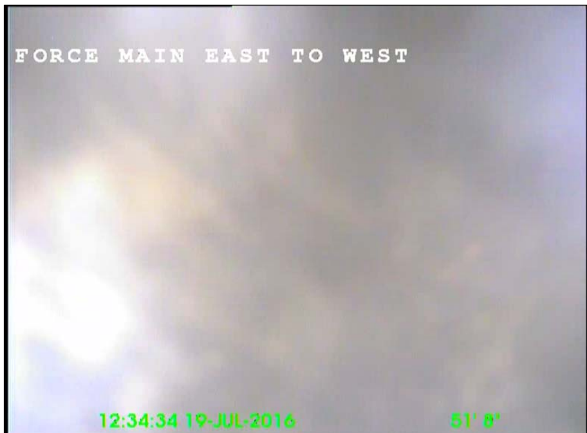
Photo: 1_1_7_A.jpg 51.8FT, Water Level, 40 %of cross sectional area
