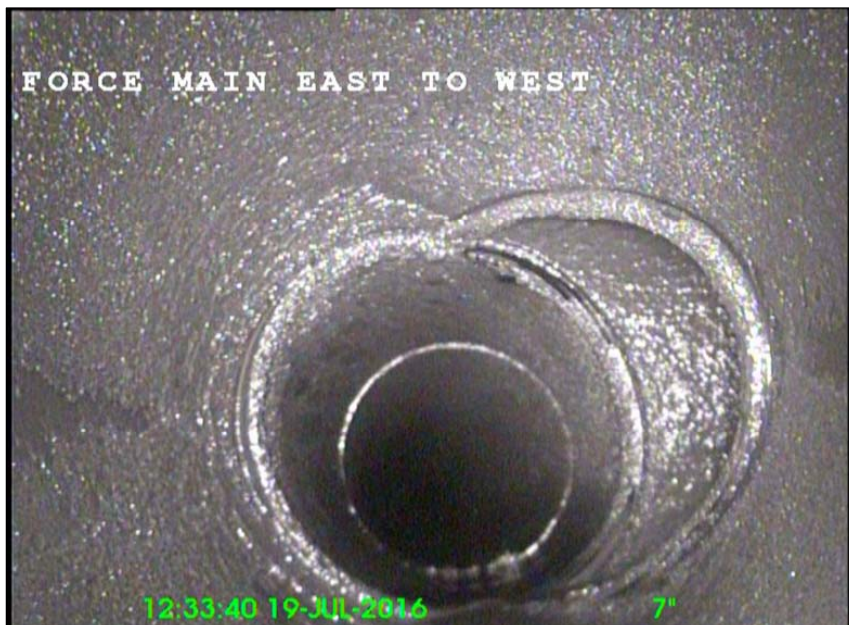
Photo: 1_1_4_A.jpg 2.3FT, Tap Factory Made, at 03 o'clock, -, within 8 inches of joint: YES, 4"
